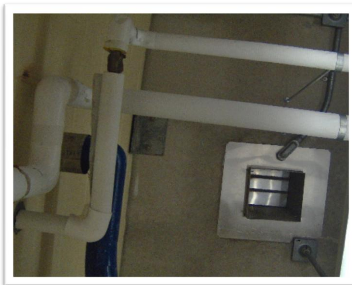
(local vent in process area)
