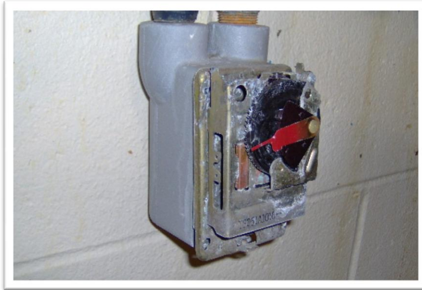
(corrosive thermostat, as noted above)
